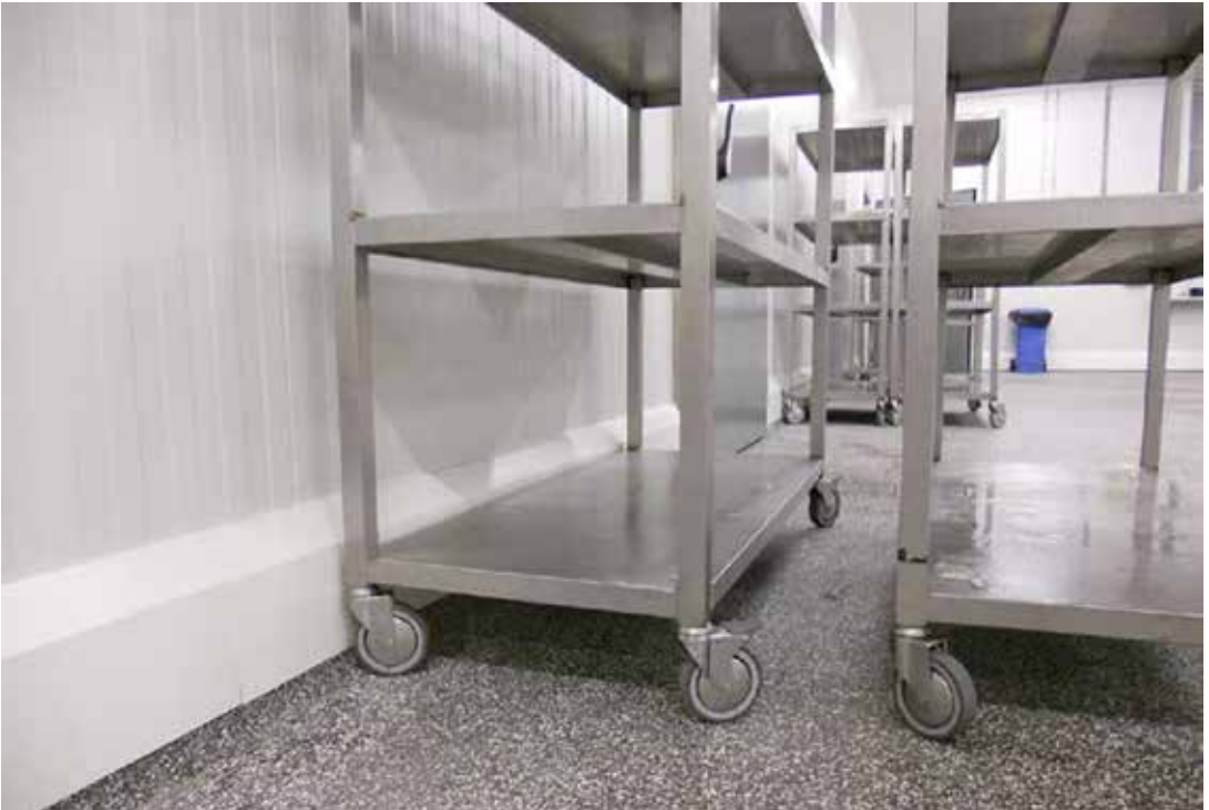
Figure 8. Kerbs with a bevelled top edge and covered at wall-floor junction (EHEDG, 2014).
