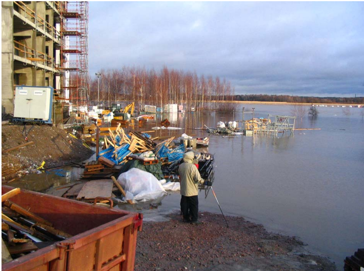
Figure 3 Construction site in the Arabianranta residential area of Helsinki during the storm surge-driven record sea-level rise of 9 January 2005 (Photo: Samuli Lehtonen).
