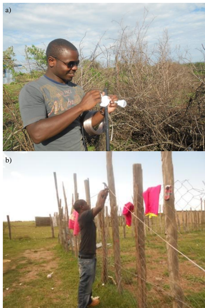
Figure 1. Installing LED lights at a boma: (a) fixing bulbs to a pole, (b) fixing a boma with connecting wires
